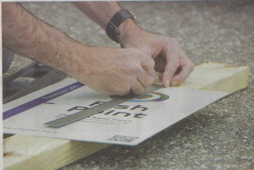
Steuben artist JT Bullitt takes measurements in preparation for installing a new Downeast Rapid Transit station sign at Fish Point in Milbridge last week. Photos by Johanna S. Billings
